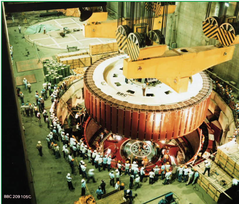
figure 11. One of the first hydroelectric generators installed in the Itaipu hydro-power plant, 1984. Half of the generating units operate at 50 Hz, and the other half operate at 60 Hz (photo courtesy of ABB Switzerland).
